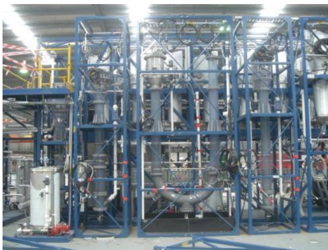
Figure 4: Resin-In-Pulp Pilot Plant
